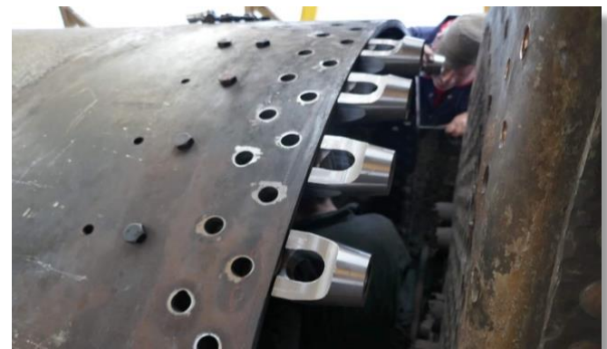
Palm stays machined and trial fitted alongside the throat plate rivet holes. (The boiler is upside down at the moment).
