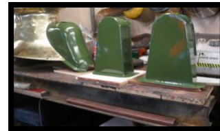
The rocking shaft covers have now been made on site, sitting alongside the brass bonnet.
