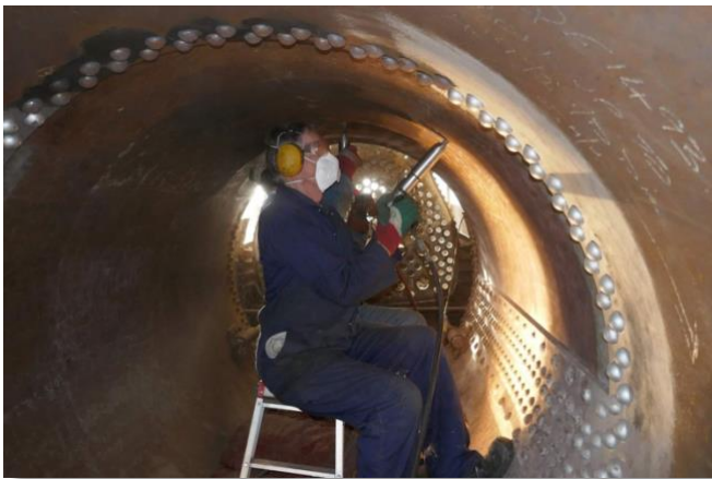
Needle gunning the inside of the boiler barrel. Very noisy and dusty work. Our extraction fan is just out of the picture.
