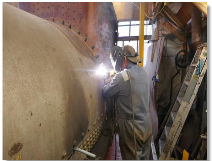
Our specialist coded welder Steve Casey, welds the lower edges of the throat plate to the main boiler. This high standard of welding is required by the boiler inspector!
