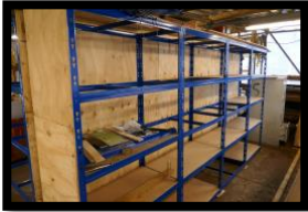
New racking being installed in our bunko booth. We're always busy improving things.
