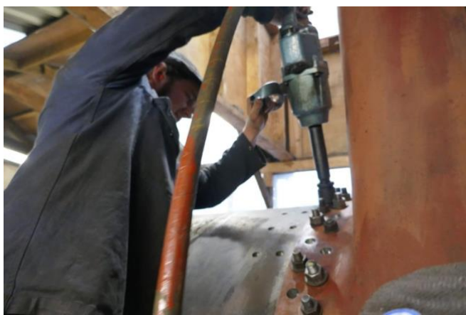
Henry tightens down the temporary holding bolts after the rivet holes are reamed to the correct size.
