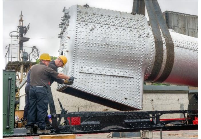
As the boiler is slowly lowered into the frames, everyone is holding their breath that it will fit into the smokebox.
