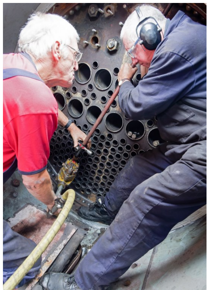
Above: Dick and TV Star Dave, use the air drill for the locating holes.
