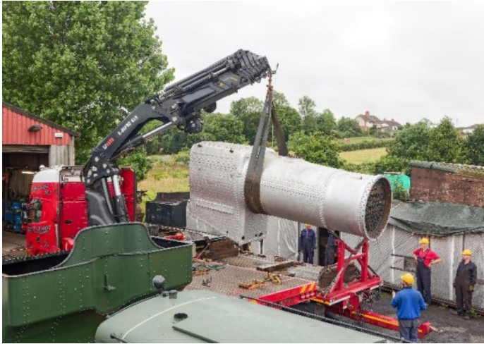
Utilising the HIAB of our transport company, the boiler is lifted across the yard to be mated with the smokebox on 4253.
