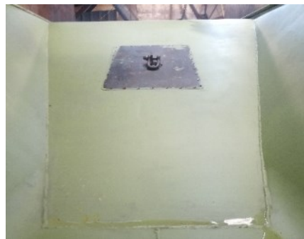
New inspection hatch fitted ( the slope is not as steep as it appears here ).
